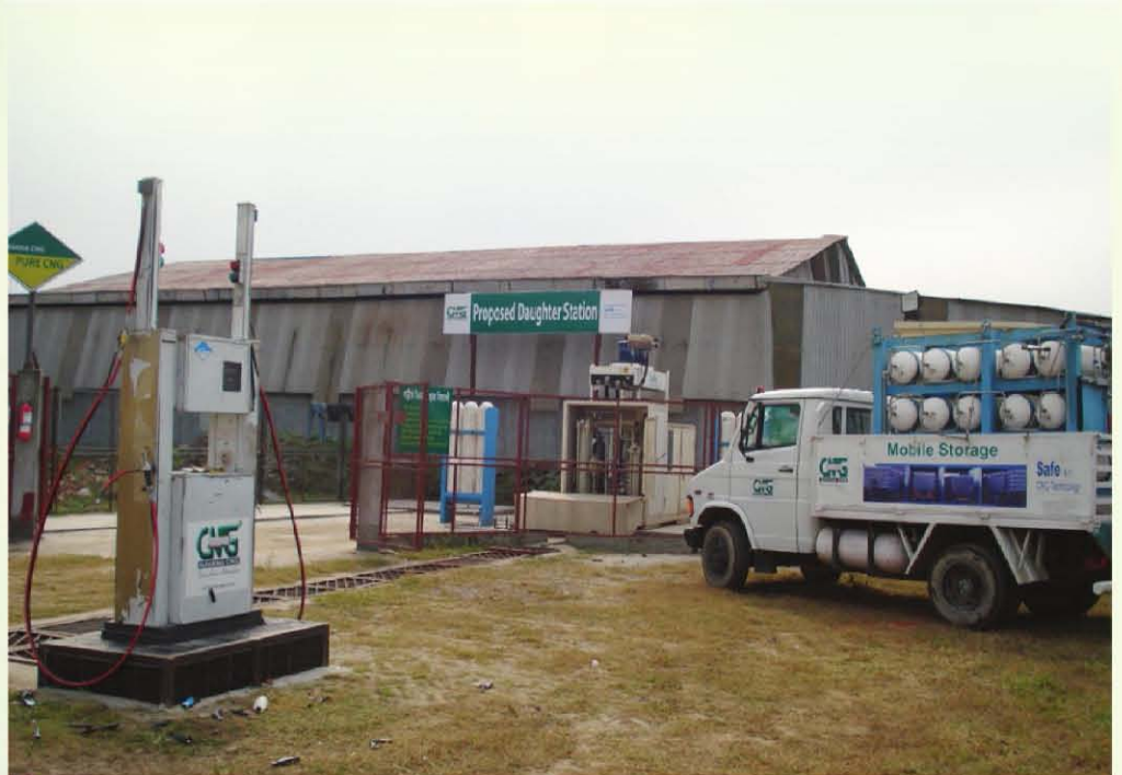
Mobile CNG Re-fueling Station
